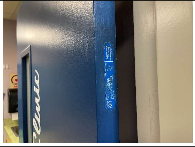
Photo 10: HM-I: Fire-rated Door Insulation, Blue Tag with Silver Lettering
